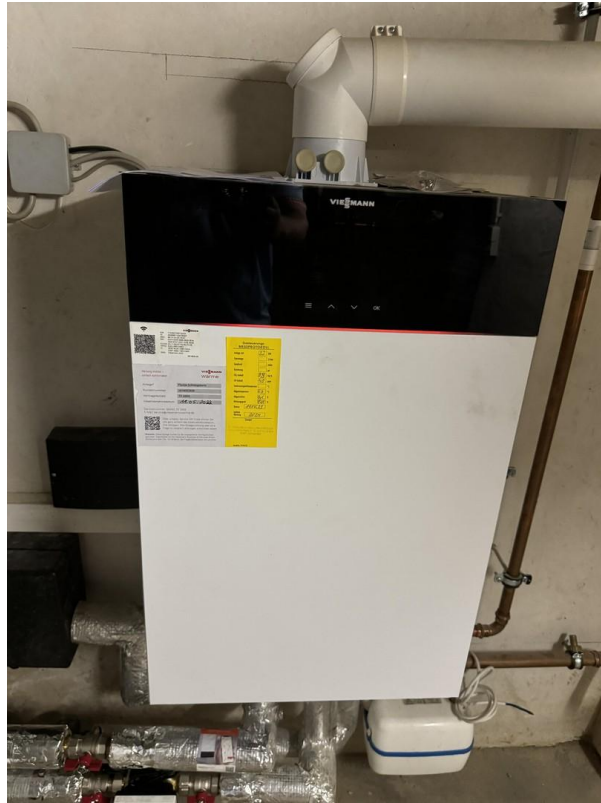
HEIZANLAGE GASS FIESSMANN
