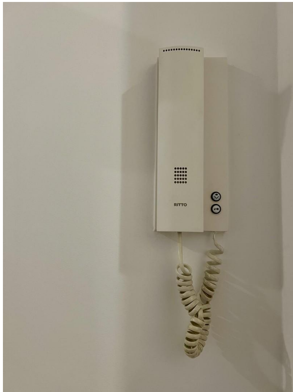
Secured intercom access
