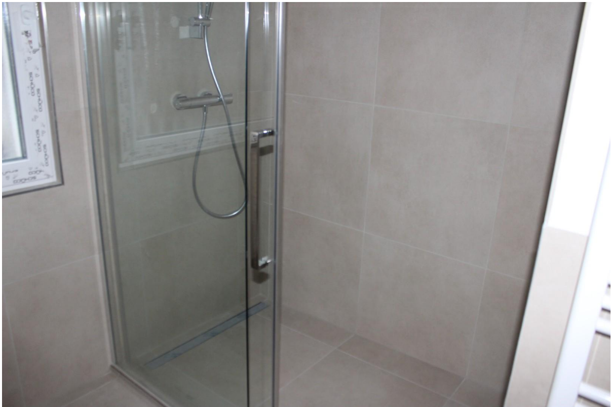
Dusche in xxl
