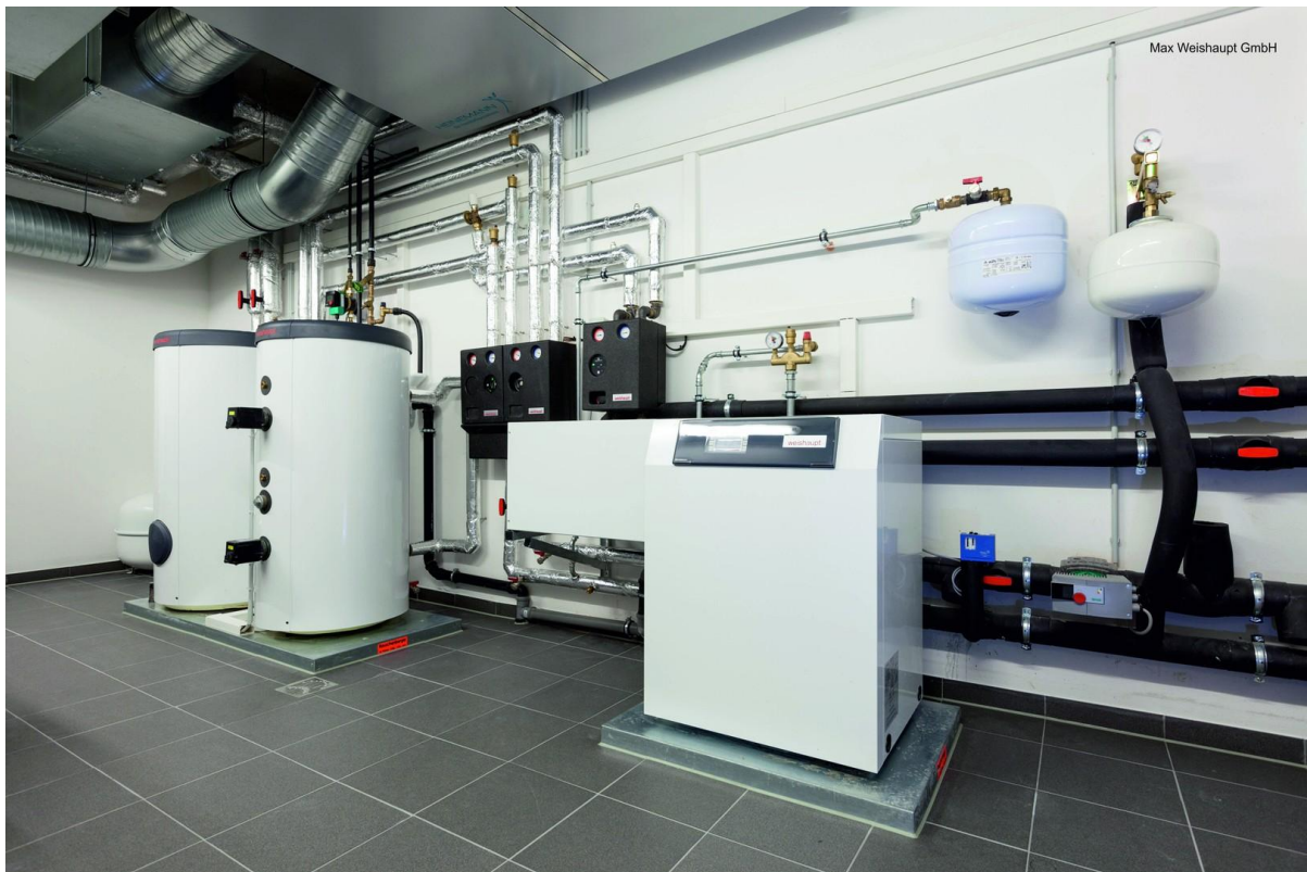
Heiztechnik - Sole WP
