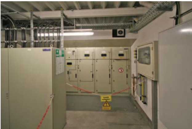
TRAFO-STATION BLOCK III
