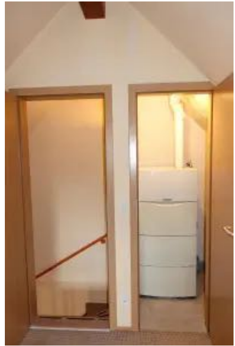
View from the window room „Dachstudio“ to the exit / central heating room
