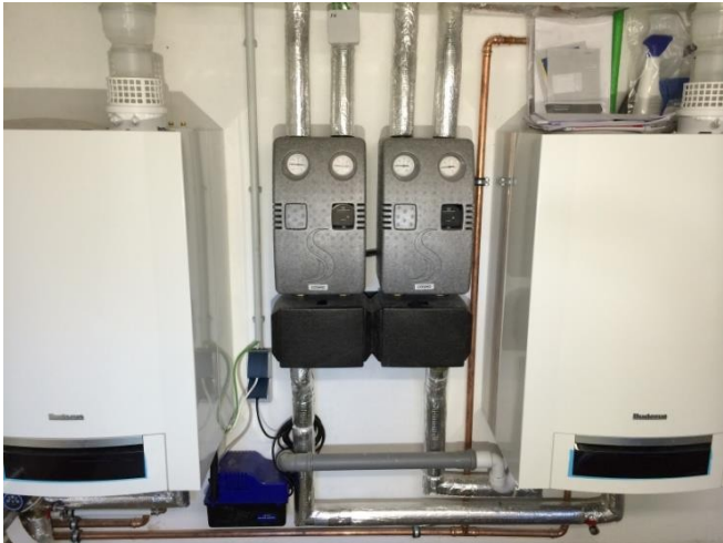
Each flat has a separate heating system
