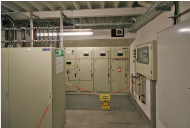
TRAFO-STATION BLOCK III
