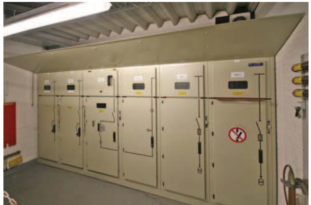
TRAFO-STATION BLOCK III
